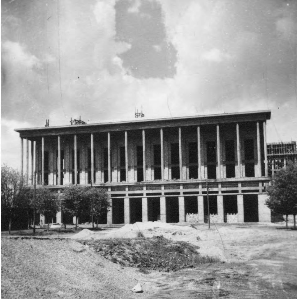
Figure 39. Construction of the Great Theater started in 1949, ca. 1950, author: unknown (Miastograf.pl digital collection).
